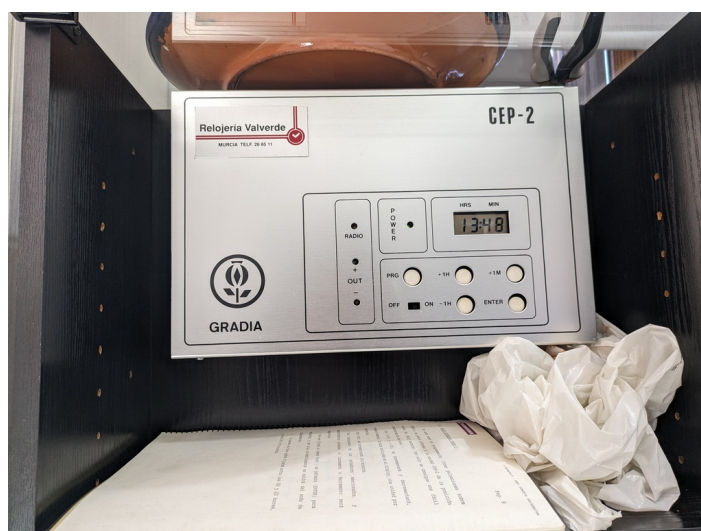
Central horaria GRADIA CEP - 2
